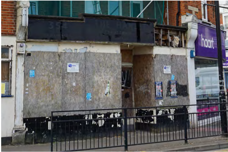
Original shop front surviving in poor condition at No.354 London Road
